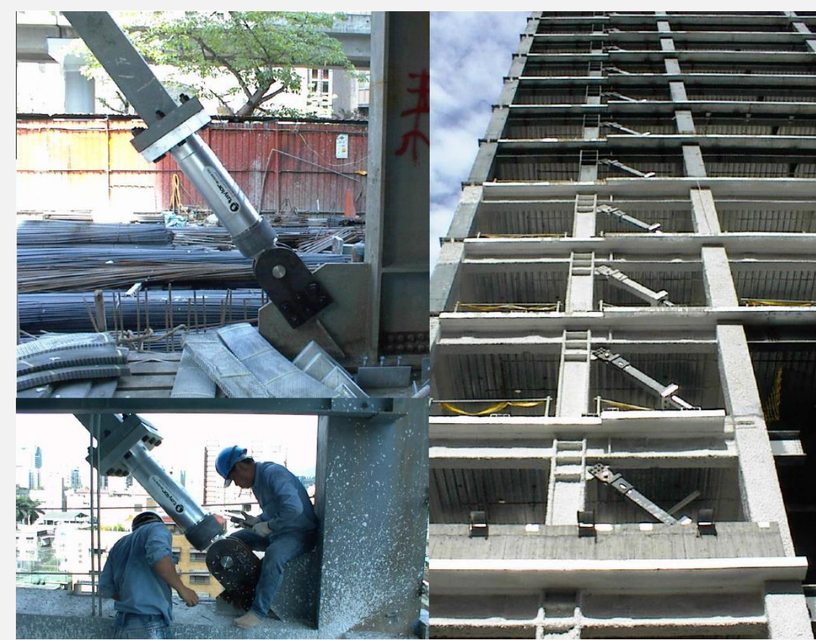
Fig.1 17-story steel structure in Taiwan equipped with 60 fluid viscous dampers (Taylor Devices India, 2016)
