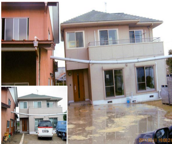
Figure 1 Tilted building after earthquake
