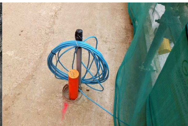
Figure 1.3.6 Inclinometer on Diaphragm Wall (September 2012)
