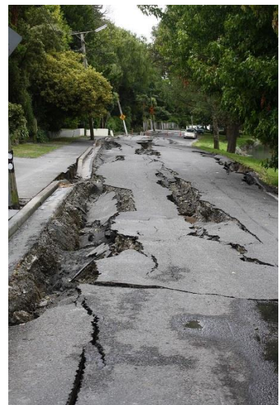
Figure 3 - Damaged Road Following 2011 Christchurch Earthquake
