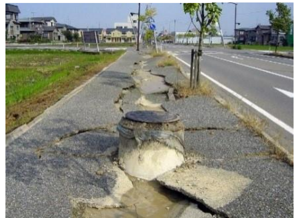
Figure 2 - Floatation of Sewer Following Soil Liquefaction during the 2004 Chuetsu Earthquake
