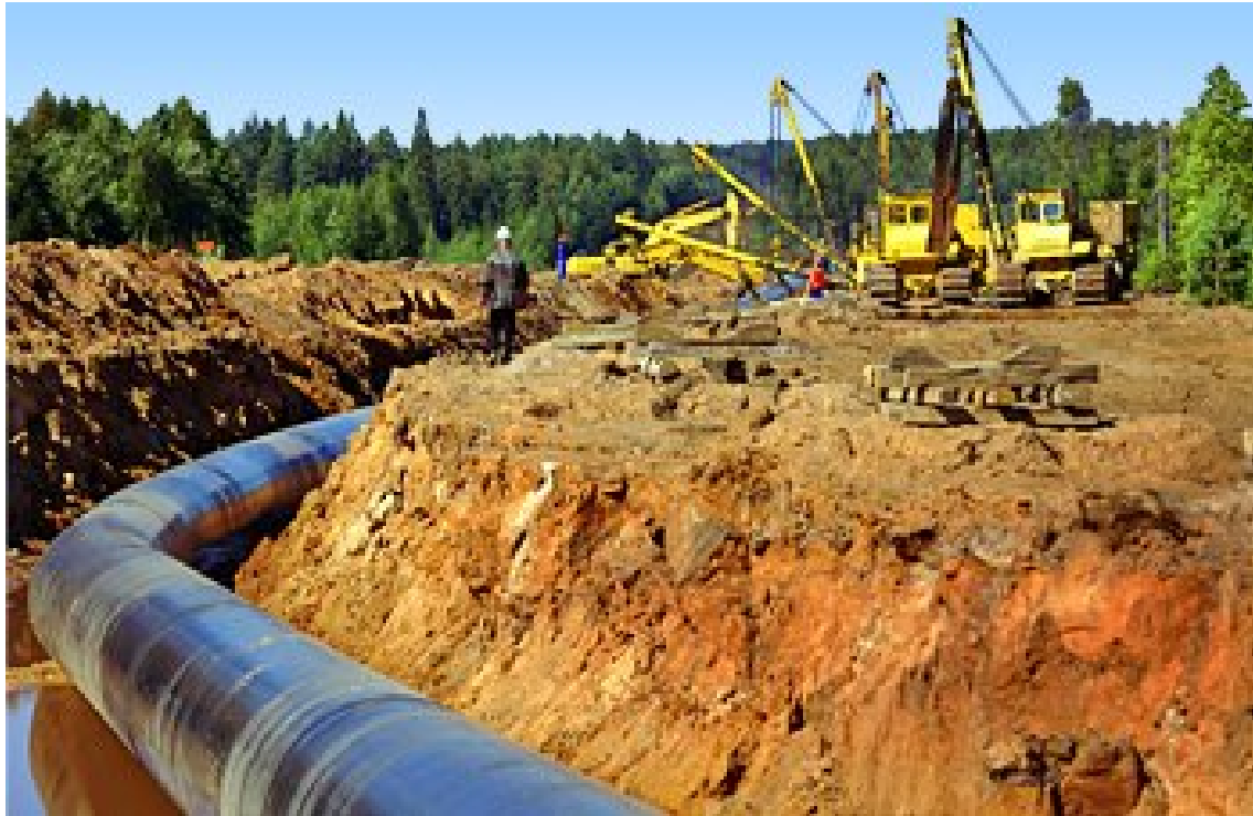
Figure 2. Underground Oil Pipeline
