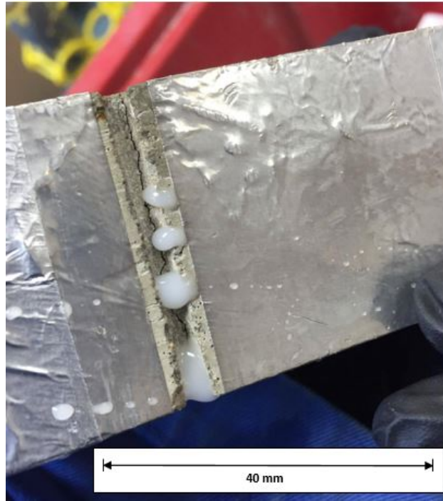
Figure 12: Injected waterproofing agent seen to have come out of the crack
