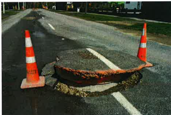
Fig. 1.1 – Uplifted pipeline in Canterbury, NZ
