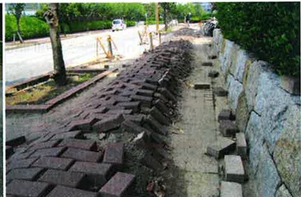
Fig. 1.2 – Uplifted pipeline in Tokyo, Japan
