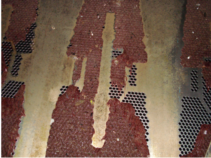
Figure 1.3: Condenser water box with blocked tube bank.
