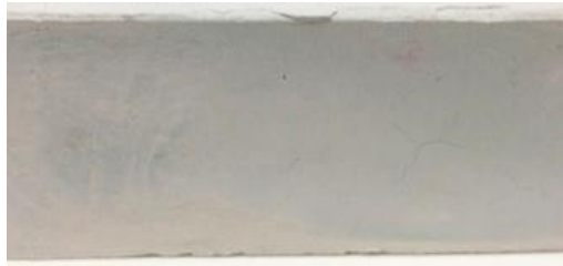
Figure 4-32 Very fine hair line surface cracking on 1-day with the addition of MgO
