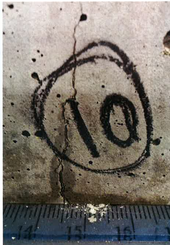
Figure 24: Little evidence was seen of new crack plane formation; the new crack is within the porous region that the low viscosity glue has filled.
