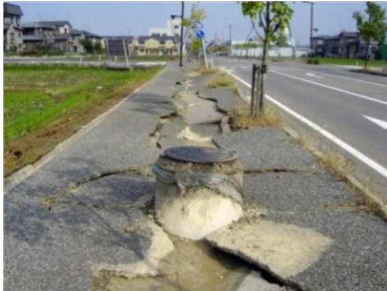
Figure 2 - Flootation of piping and inspection cover - Chuetsu, Japan 2004
