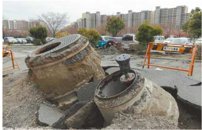
Figure 3 - Flootation of underground storage tanks - Tokyo, Japan 2011
