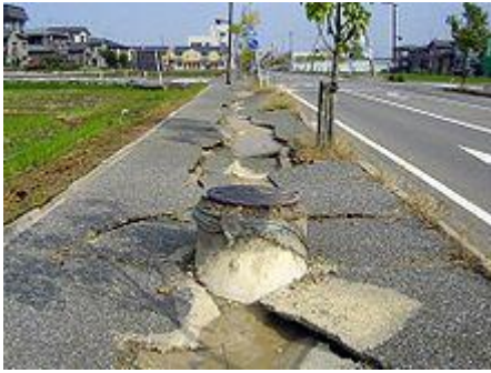
Fig. 1.2 - Differential Structural Settlements following Liquefaction
