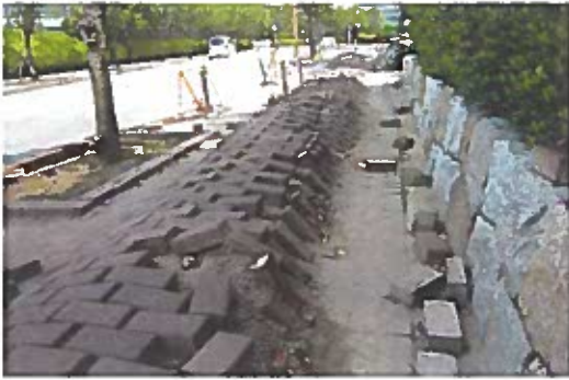
Figure 1: Uplift of underground utility in Chiba (Tokyo metro) area (Structural Engineers Association of Washington, 2011)
