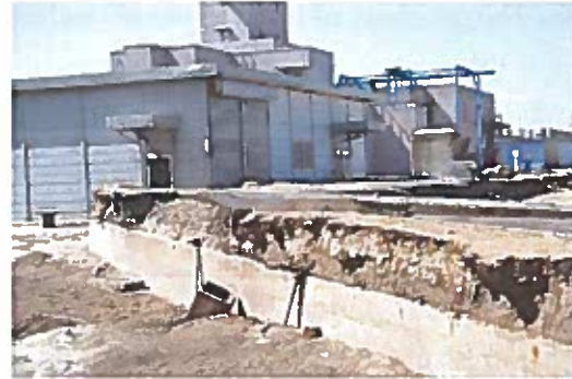
Figure 2: Uplift of utility conduit at water purification plant in Kamisu city, Ibaraki Prefecture (Tokimatsu et al., 2013)
