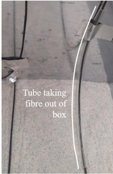
Figure 14: Fibre running via a tube out of the box.
