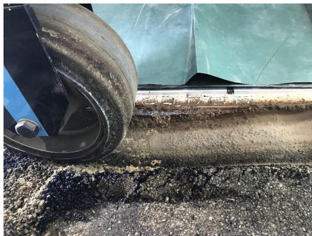
Figure 34 - Surface rutting present at the end of test 7
